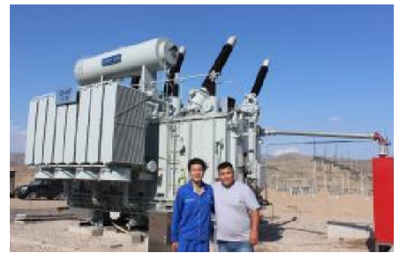
161kV 15Mvar Reactor to SECL , Canada
