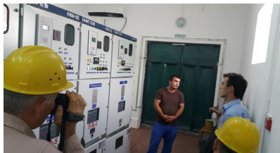
Vaheidate 110kV substation Tadjhikistan
