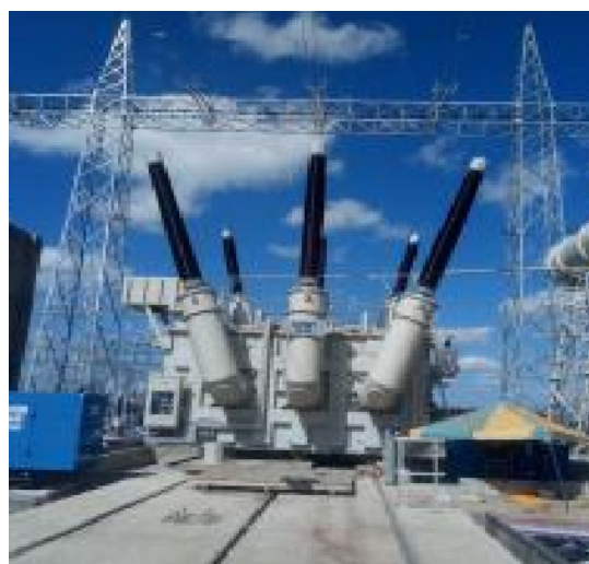
400kV 200MVA Transformer to KETRACO-Kenya
