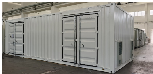
Singapore 200MW BESS Project
