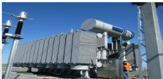
115kV 90MVA Transformer to First Quantum Minerals, Finland
