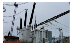
400kV 300MVA ,Power transformer to CGES , Monre negro
