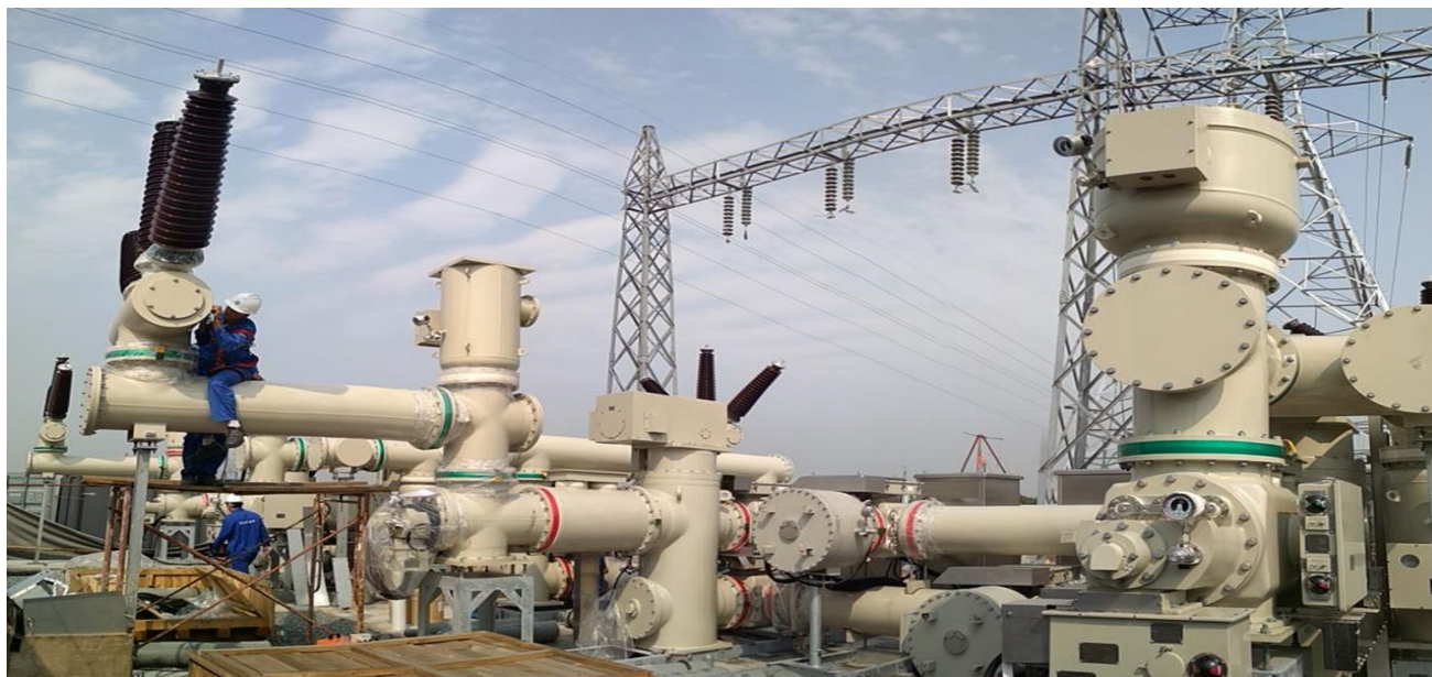
110kV GIS at Allinder Substation in Nederland
