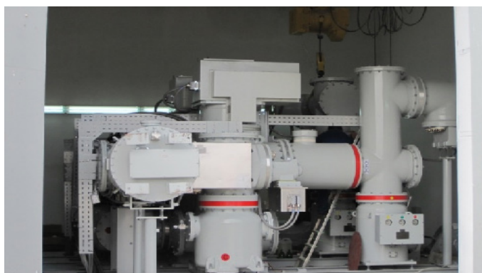
145kV GIS in Ukraine international airport
