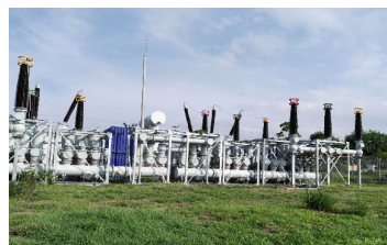
252kV GIS Panama project
