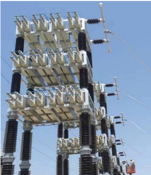
Afghanistan 220 kV Outdoor Capacitor Complete Plant Project TBB220-40000/346-BLW
