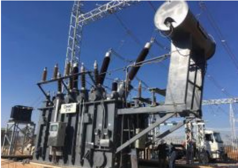
220kV 125MVA transformer to BPC, Botswana
