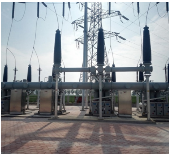
252kV GIS in Dalian Solar project
