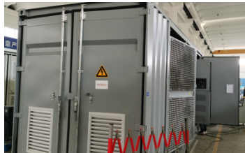
Nigeria KANO Solar Farm Project
