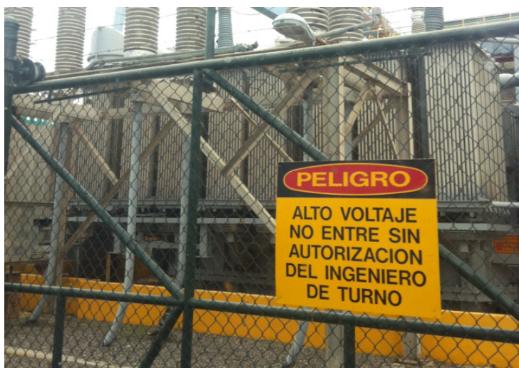
230kV 570MVA Step-up Generator Transformer in Puerto Rico
