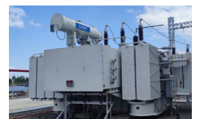
Philippine Nexif Energy CARE 75MW Solar Power Plant
