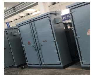
G2E 33kV0.4kV 4MVA Power Transformer Project
