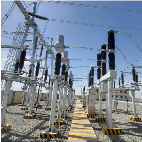
Aksey 100MW Solar Project
