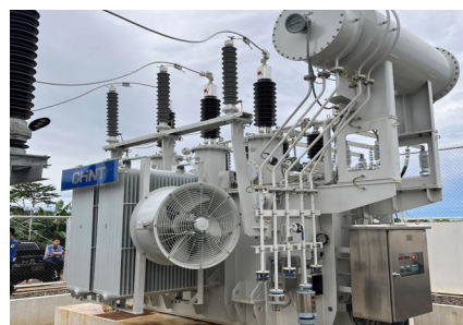
Philippine PAVI GREEN 20MW Orion Solar Plant
