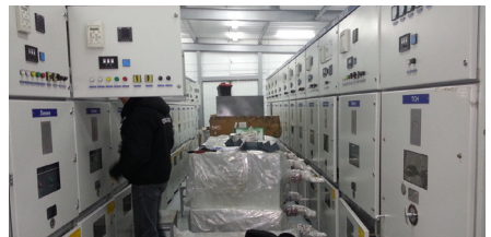
AK Altynalmas substation Kazakhstan
