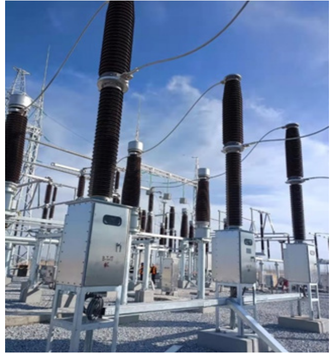
Uzbekistan Navoi solar plant project
