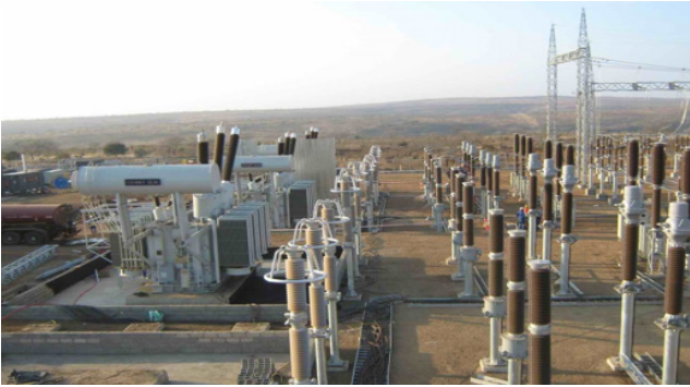
Aggreko(UK) Mozambique 275kV step-up substation
