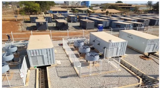
Tanzania Voltage drop compensation project for Buly Gold Mine project ZTSVG-C15/6.6-O-W
