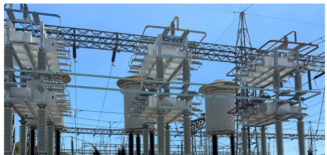
Philippine NGCP Compostela Substation
