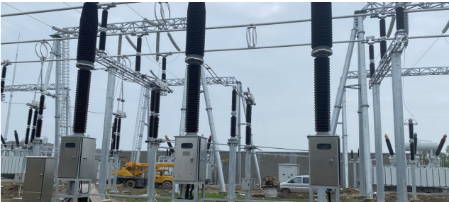
Tanzania 220kV Substation
