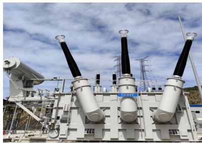
400kV 300MVA ,Power transformer to CGES , Monre negro
