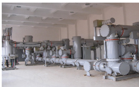
145kV GIS in Angola
