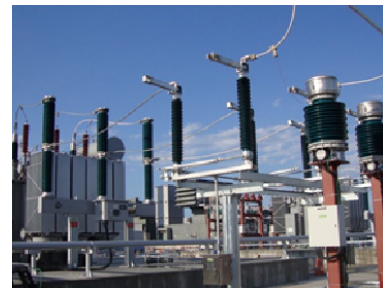
66kV AIS at TEPCO substation in Japan
