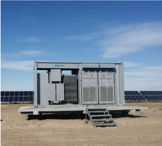
Kazakhstan 100MW solar power project
