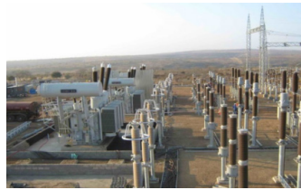
Aggreko(UK) Mozambique 275kV step-up substation
