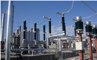
66kV AIS at TEPCO substation in Japan
