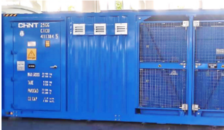
Philippine Data Center Project
