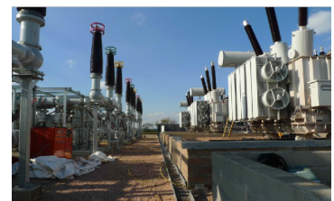
252kV GIS In Philippine
