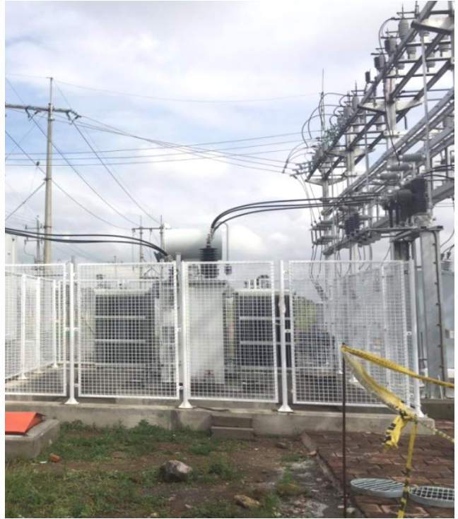
Mexico Power Plant Project ZTSVG-C3/23T-O-W
