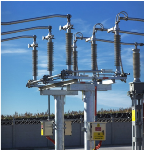
Wind power plant in Romania
